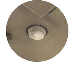
4. LED interior lighting
